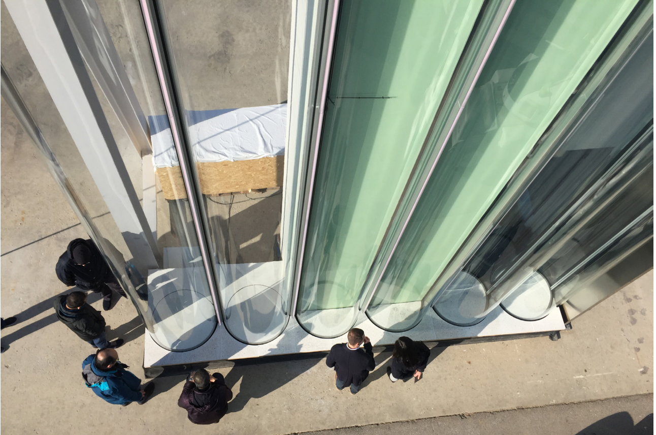
Top: Performance facade mock-up of aluminium stick system overclad with bronze panels
